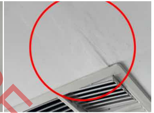
Cracking along sheet joint
